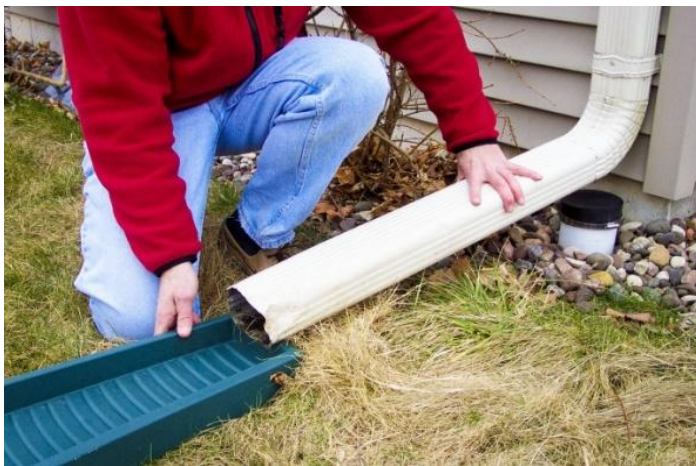
Picture of a disconnected downspout
